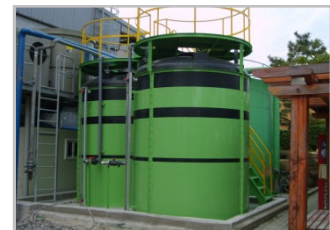
· Wastewater Treatment Facility
