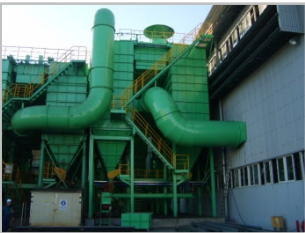
• Air pollution control equipments
